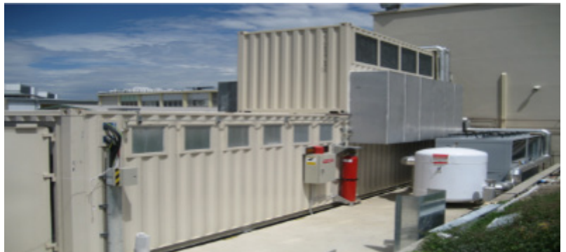
Schneider Electric modular data center installed at Animal Logic Animation Studio in Sydney, Australia.
