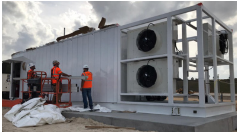
Modular data center installation for grocery retail and delivery business.
